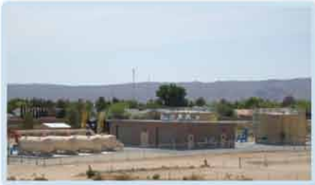
Arsenic removal facility located at Well 13 near Mahan St. and Felspar Ave. treats water from both wells 11 and 13.
