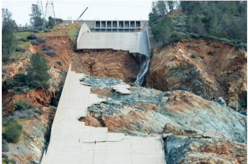
Figure 4-23. Oroville Dam Spillway after 2017 failure.
